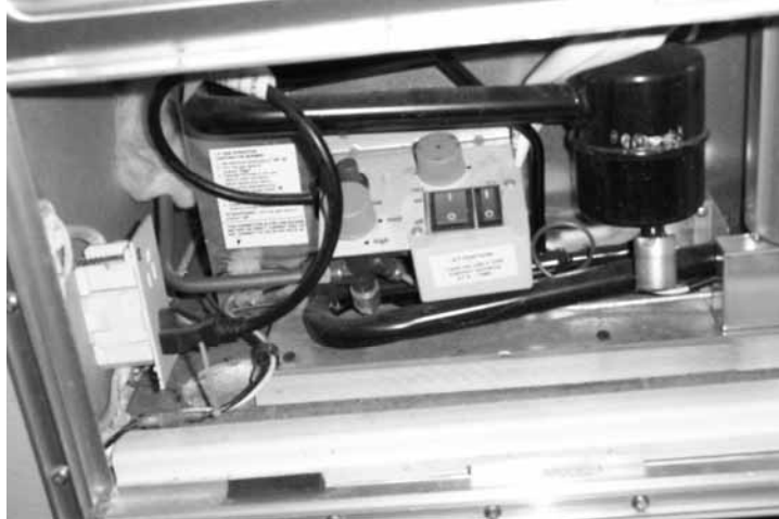
Refrigerator controls in ventilated compartment on street side of unit.
